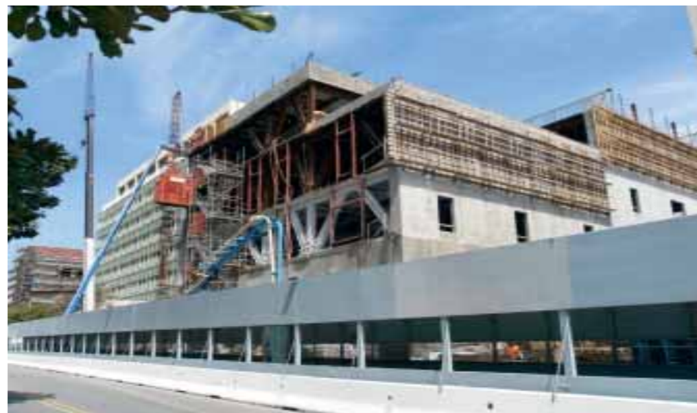
The new Nethercutt Emergency Center will be housed on the ground level of the Southwest Wing, being built on 15th Street near Arizona Avenue.
